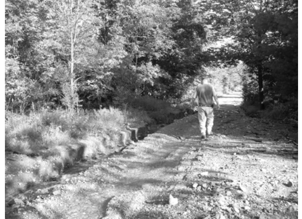
Daryl Burlett inspects damage on North Stage Road.
